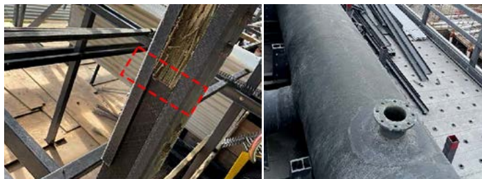
Figure 10: Missing Bearing Plate (left), Uninstalled Standpipe (right)
