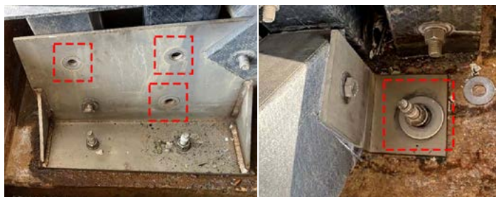
Figure 9: Missing Hardware on Base Anchor (left), Undersized Anchor Bolt (right)
