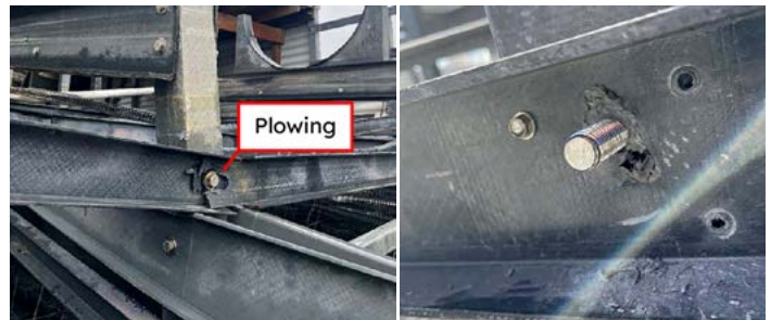
Figure 14: Hot Water Basin Joist Exhibiting Plowing (left), Missing Hardware & Plowing of Member (right).
