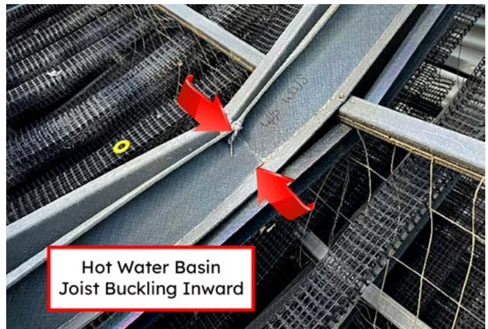
Figure 15: Hot Water Basin Joist Buckling Inward.
