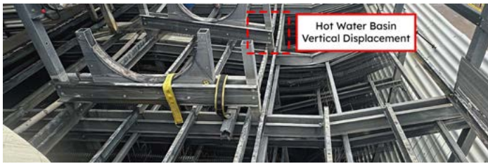
Figure 16: Hot Water Basin Supports Vertical Displacement.
